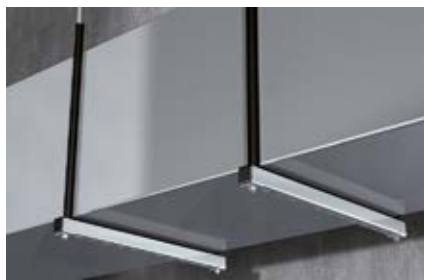
Air duct with Hangszigetelés on installation channel
